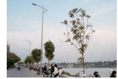
LED street lighting system with wireless network control, 3 MinebeaMitsumi, Cambodia
