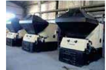
High-efficiency Heat only Boilers, Suuri-Keikaku, Mongolia
