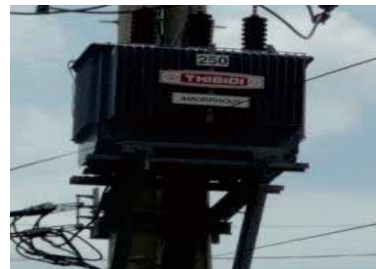
Amorphous transformers in power distribution, Hitachi Materials, Vietnam
