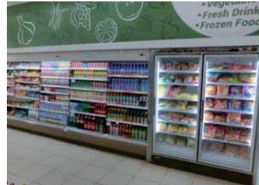
Energy saving at convenience stores, Panasonic, Indonesia
