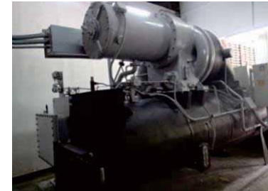
High efficiency air-conditioning and process cooling, Ebara refrigeration equipment & systems, Indonesia
